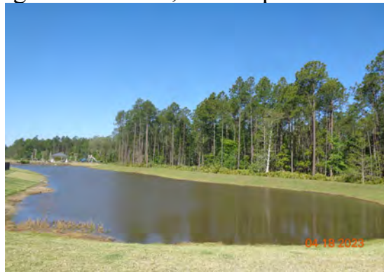
Pond XX: Pond in good condition, no algae noticed, treated perimeter weeds.
